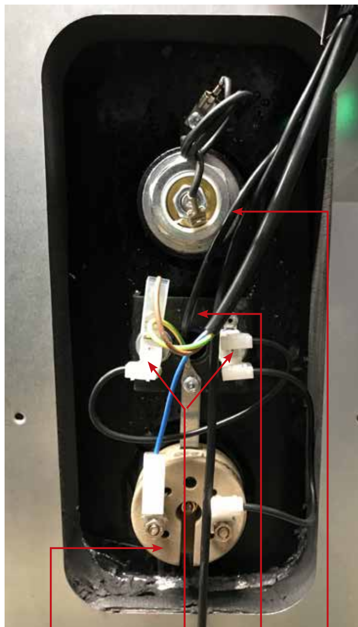
Electrical water heater
